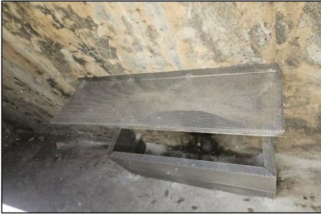
Installed Connector Pipe Screen (CPS-Mod)
