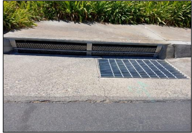
Installed Automatic Retractable Screen (ARS)
