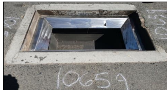
Installed Grate Inlet Screen (GITS)
