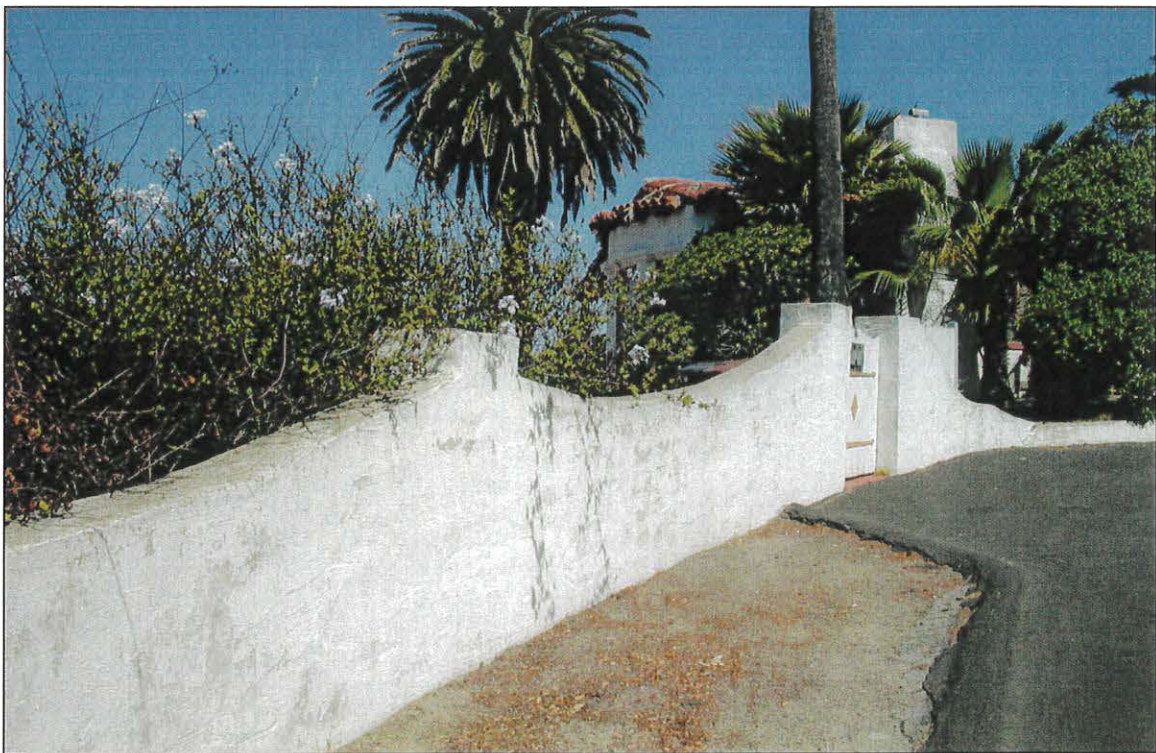
Photograph 12: Subject property, east retaining wall (foreground) and existing residence (background), view northwest, 2002 (CA)
