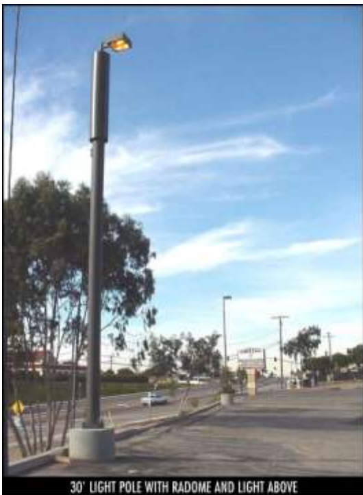
30' LIGHT POLE WITH RADOME AND LIGHT ABOVE
