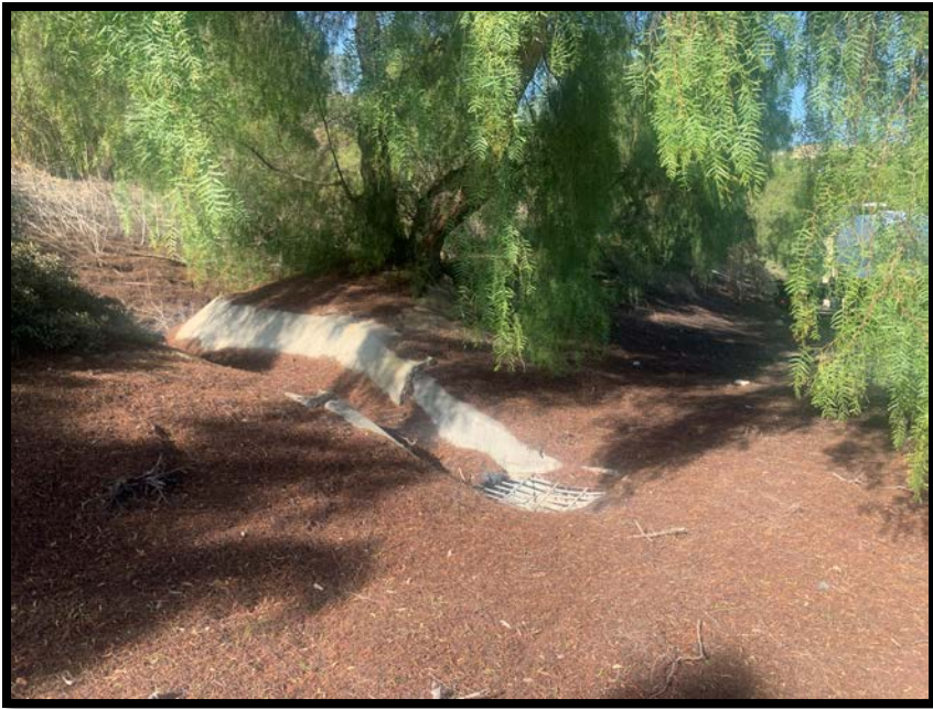
Photo 5: Ribbon drain located in the western segment of the BSA. Photo date: November 4, 2022.
