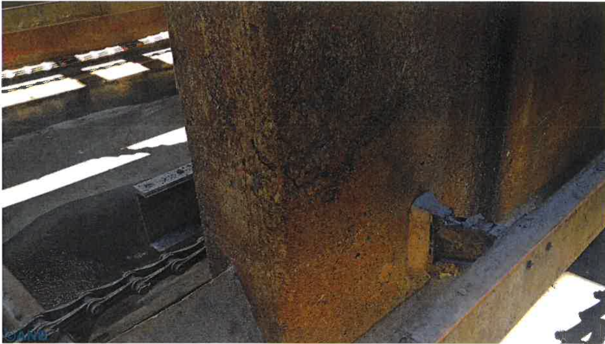
Figure 3: Large surface spalls at interior walls corners
