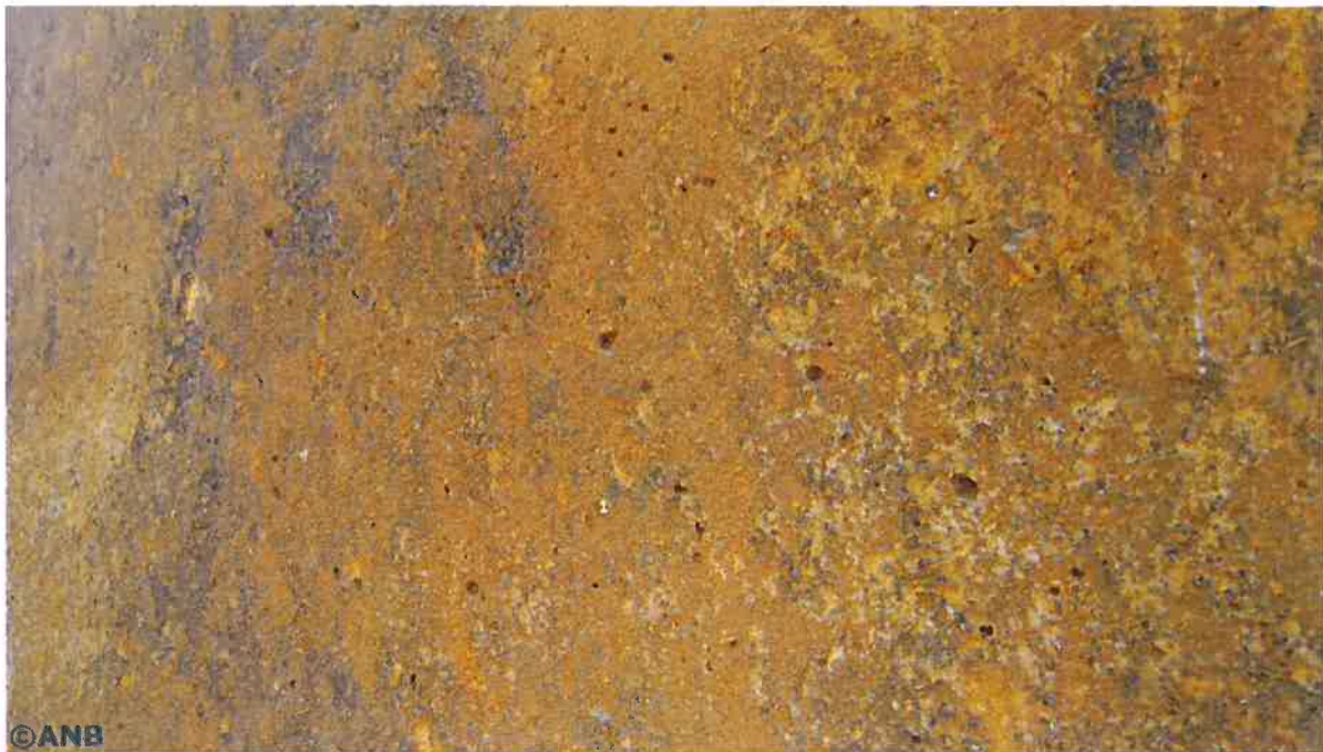
Figure 1: Concrete pinholes throughout interior wall surfaces
