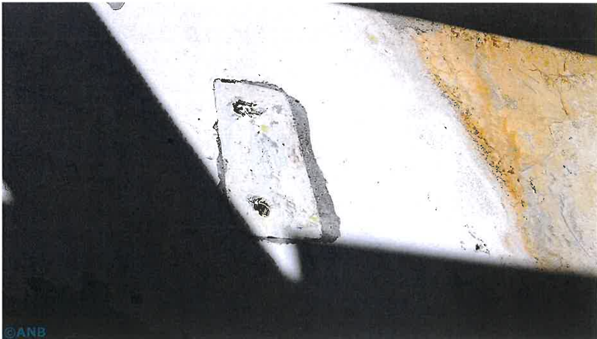
Figure 6: Abandoned steel bolts on walls throughout
