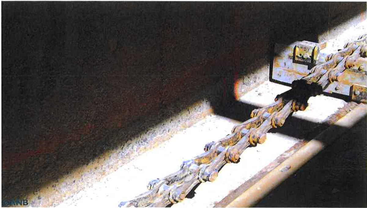
Figure 7: Wall bottoms worn out by scraping solids at mixing blades.
