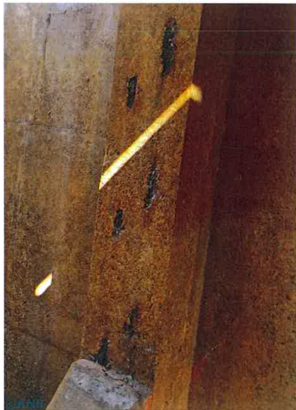
Figure 8: Rusted reinforcement at prior concrete cuts.
