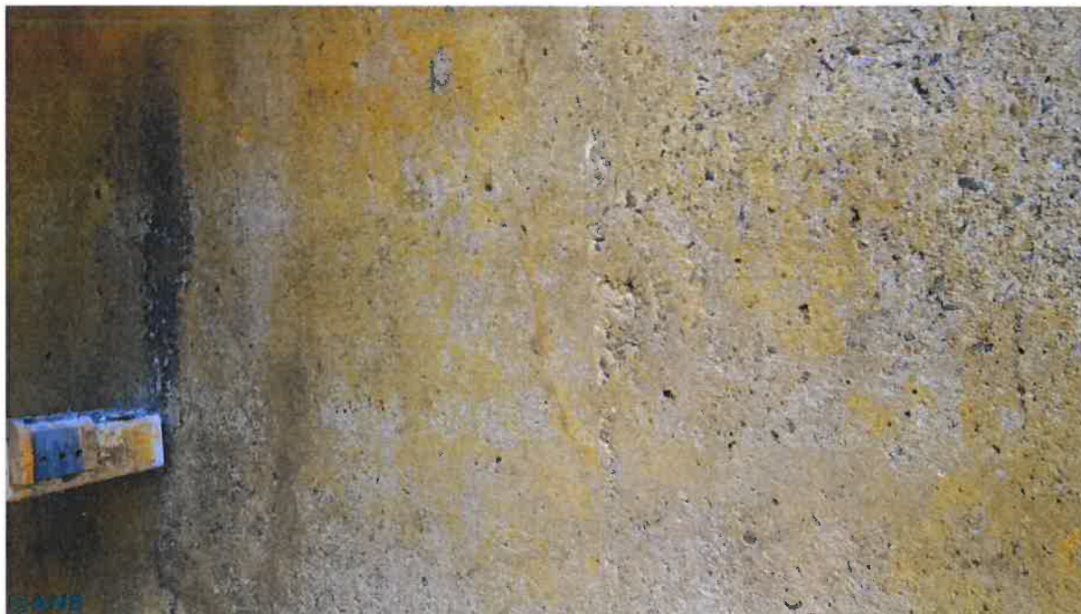
Figure 2: Small surface spalls throughout interior wall surfaces
