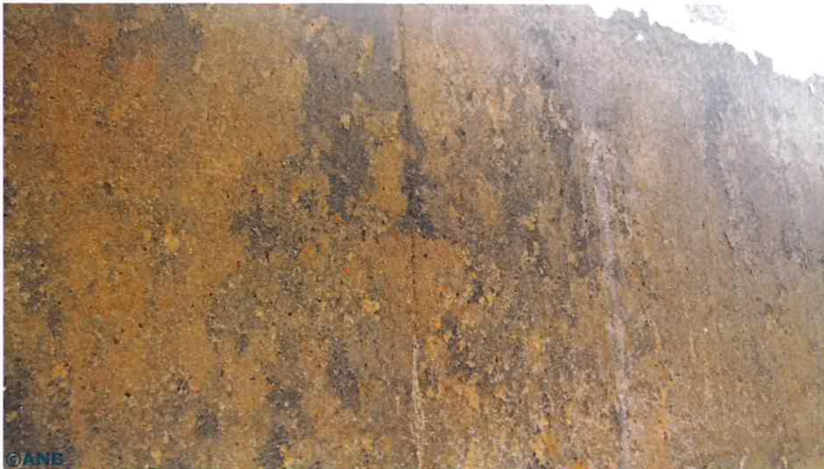
Figure 4: Vertical wall cracks at construction joints
