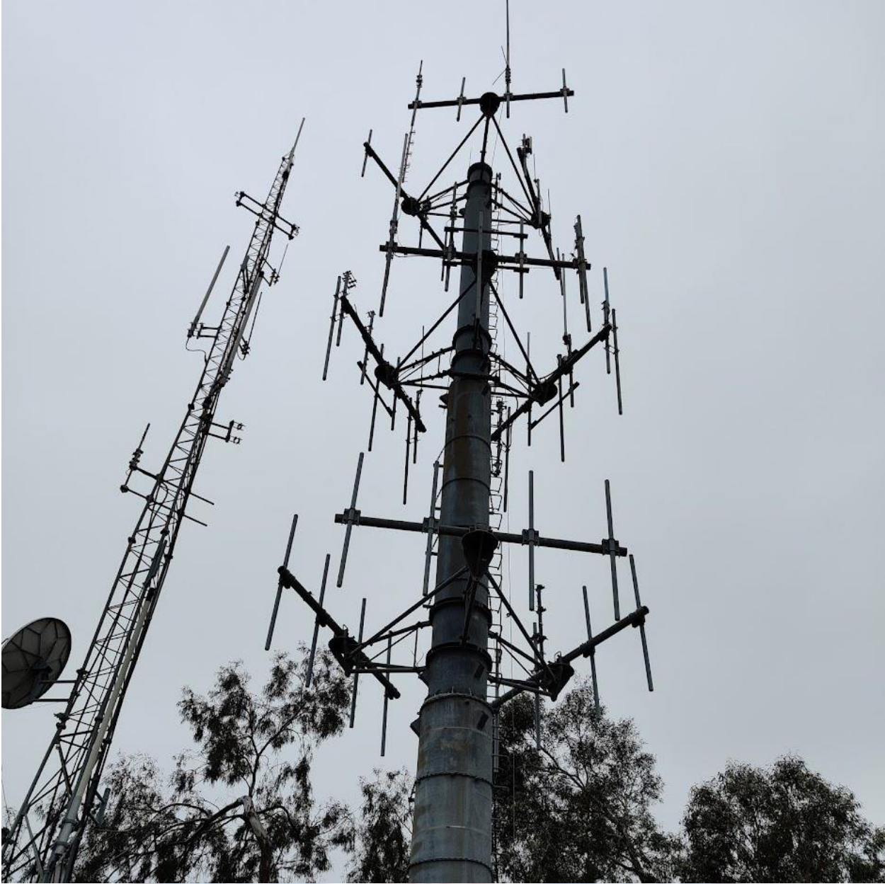
Antenna tower at San Clemente Summit
