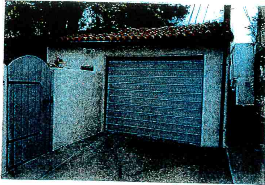
Single Garage with failing garage door (probably not original). Interior Workshop space to the left has separate entry door from patio.
