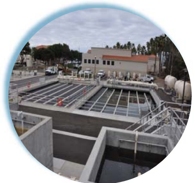
Water Reclamation Plant
