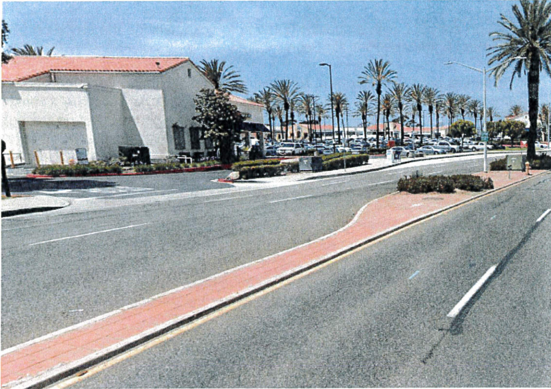
Photo 1. Existing red stamped concrete to be removed, and low concrete curb to be replaced with new full height concrete curb.
