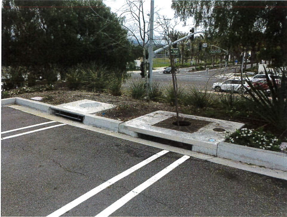
SEWER DRAINS ON SITE, CORNER OF TARGET AND AVE. VISTA HERMOSA
