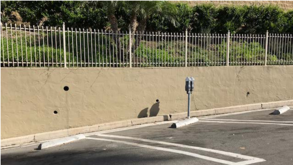
View of block wall and wrought iron fence from the City's Parking lot.
