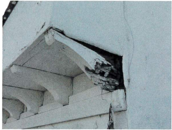
Image 5-4: Damage at decorative wood corbel. 2013.
