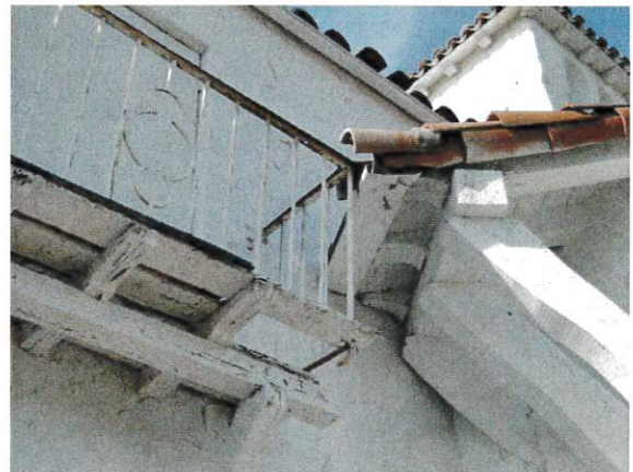
Image 5-3: Damage at decorative balcony. 2013.
