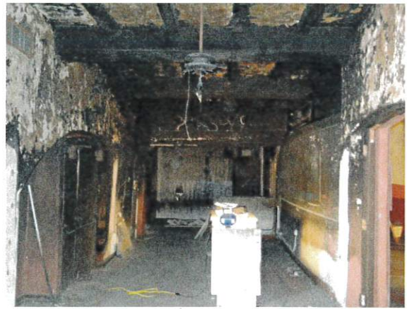
Image 5-10: Damage from a 2005 fire in the Lobby. 2013.
