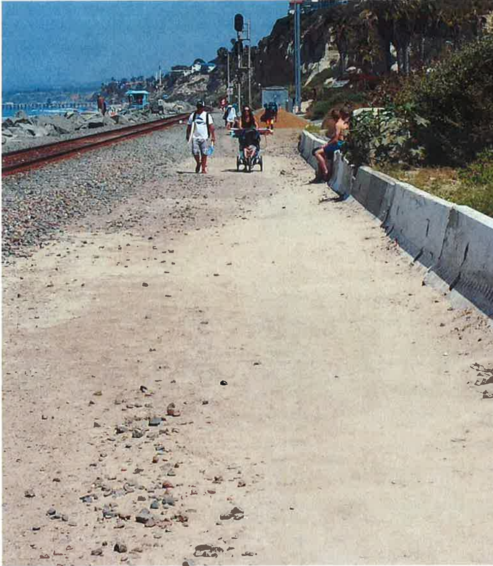
Photo 5: This photo demonstrates the jagged, golfball-sized rocks stabilizing the railbed, which creates a shifty surface for pedestrians and bicyclists. To protect trains from crumbling sandstone and rocks, railroad maintenance crews added temporary concrete k-rail barriers between the sandstone cliffs and the rail bed. The barriers narrowed the navigable path, safeguarding trains but increasing risks to trespassers who have been using the rail bed for decades.
