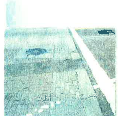
Decorative crosswalk treatments made of distinctive materials can become uneven over time (Credit: Ryan Snyder)
