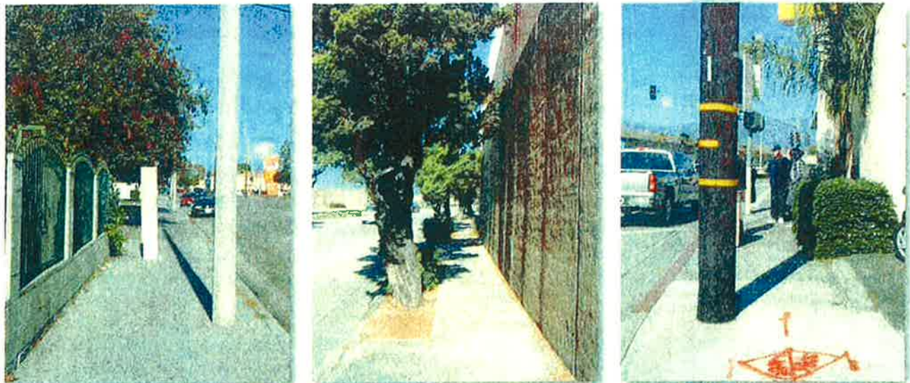
Sidewalks constructed without adequate design guidelines (Credit: Chanda Singh)
