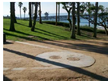
Underground unit installed at Parque Del Mar (next to Pier Bowl parking lot).
