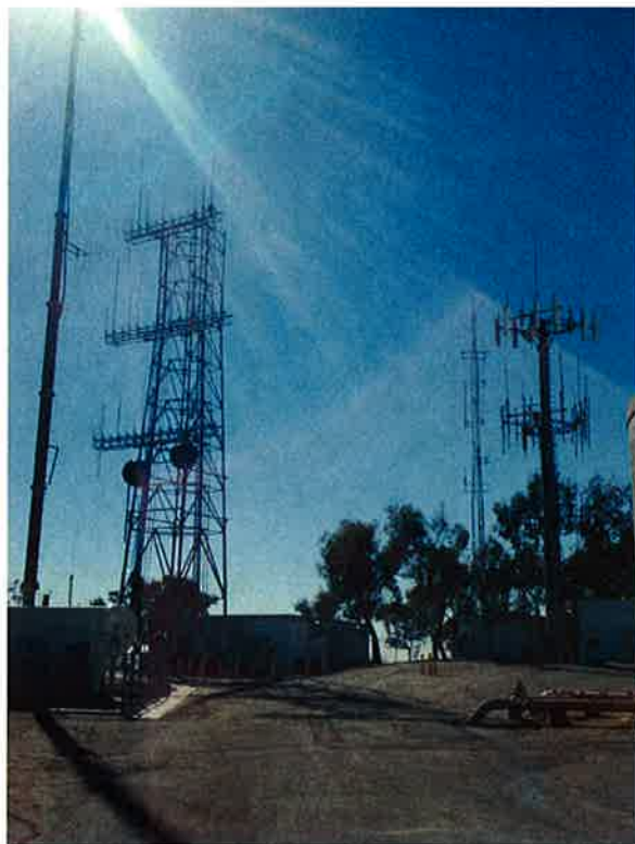
Existing Communication Facilities
