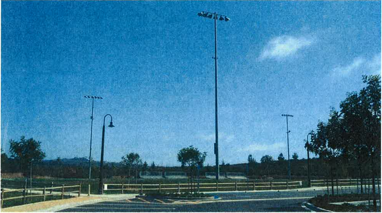
Cellular Light Pole Site (View 2).
