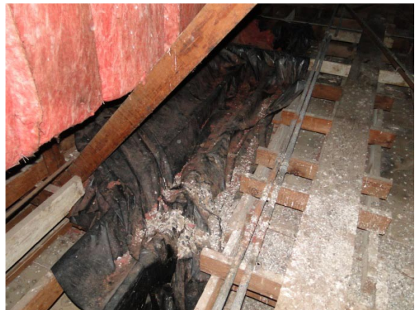
Image 5-14: Tarps used in the theatre attic space in an attempt to reduce water infiltration. 2013.
