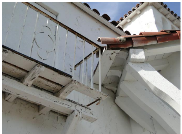
Image 5-3: Damage at decorative balcony. 2013.
