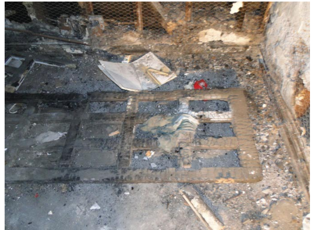
Image 5-11: Fire damaged door to act as template for reconstructed doors. 2013.
