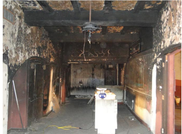
Image 5-10: Damage from a 2005 fire in the Lobby. 2013.
