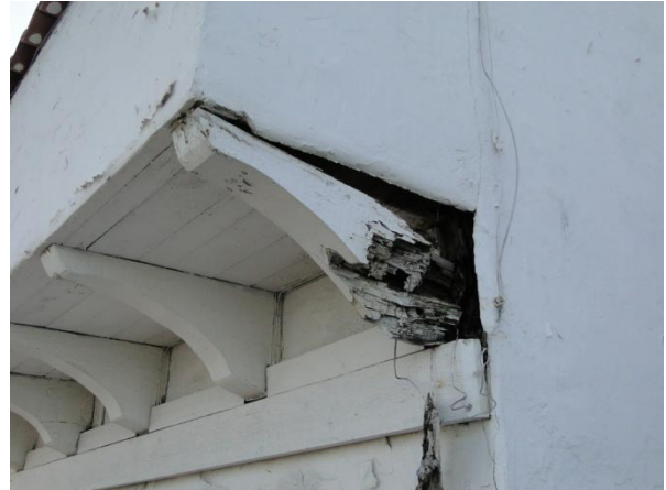
Image 5-4: Damage at decorative wood corbel. 2013.
