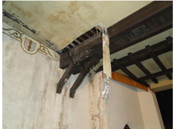
Image 5-13: Decorative box beam and concealed grill for original air conditioning system. 2012.
